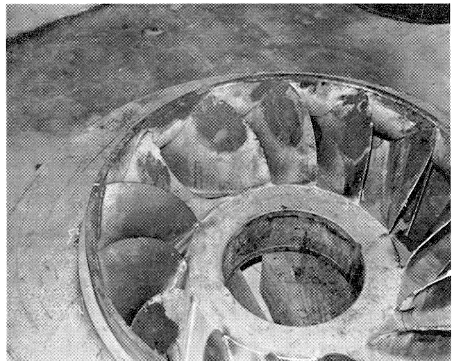
Figure 7. Closed First Stage Impeller Blade Failure Near the Leading Edge after Seven Years of Operation can be Seen at 10 O'Clock. Impact Damage is also Apparent on the Leading Edge of the Other Blades.
