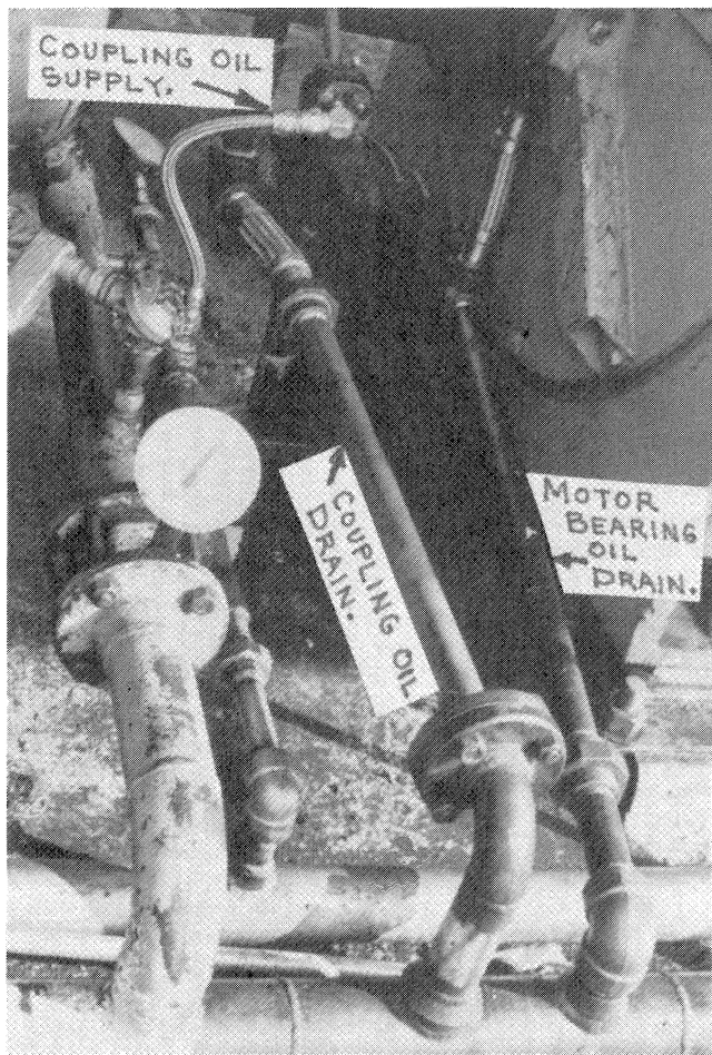
Figure 44. Motor Bearing Oil Return Lines Were Increased in Size from 3/4 in. to 1 1/4 in.
