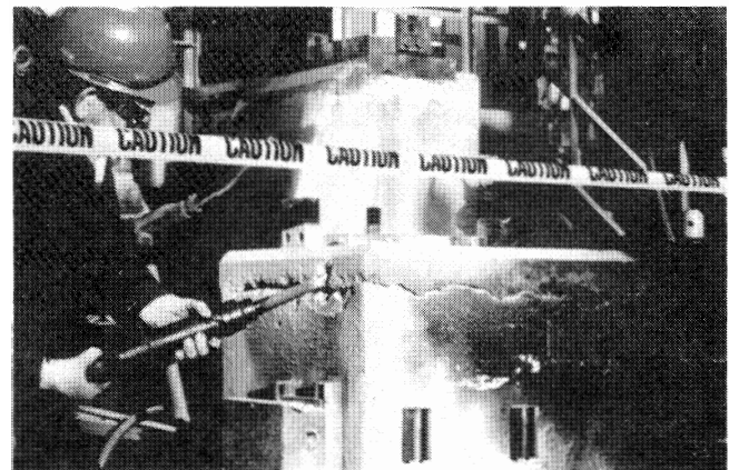
Figure 20. Chipping of Existing Grout Should Begin between the Concrete and the Grout.
