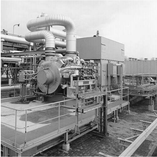
Figure 1. The Completely “Dry” Compression String at the Tjuchem Site of NAM in The Netherlands.
