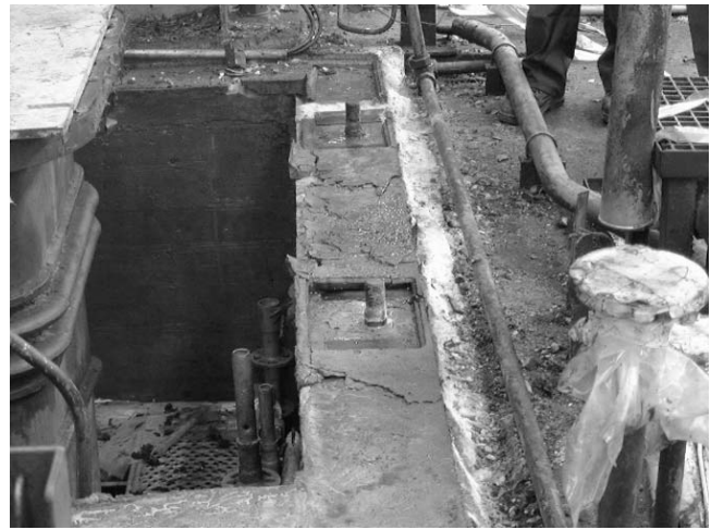
Figure 36. As-Found Deteriorated Condition of Foundation.
