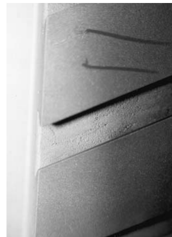
Figure 5. Corrosion Pitting in an Alloy Steel Dovetail Blade Attachment Region.
