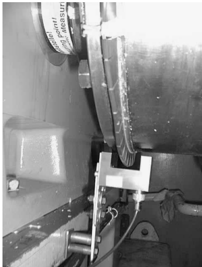
Figure 15. Installation of Strain Gauges and Telemetry-Components on Moto-Compressor for Automatic Monitoring of Load.
