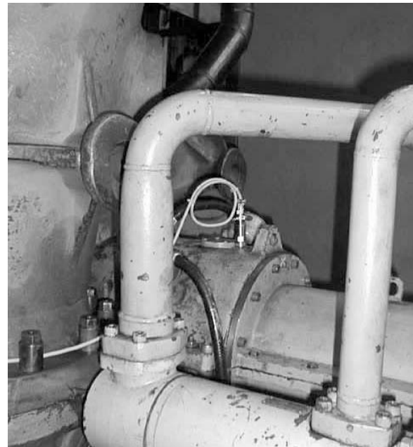
Figure 13. Arrangement of Accelerometers on DE Side Housing of Gear Unit and on Compressor DE Side Bearing Housing.
