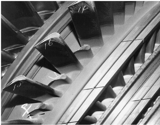
Figure 43. Five Broken Freestanding L-2 Blades Broken Off at location of Phase Transition Zone.
