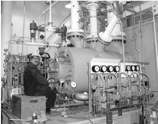
Figure 5. Platform C-12 Compressor 25MB5/61.
