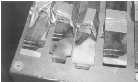
Figure 21. Wear of Sealing Plates Used Between Transition Pieces.
