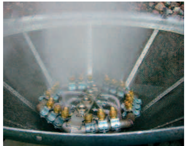
Figure 3 Water wash manifold with eight nozzles giving 75 \mu\text{m}_{\text{VMD}} droplets at 4.3 l/min
