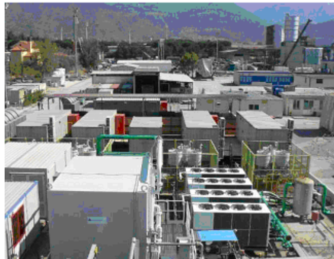
Figure 13. Full Drive System with Load Machine at Oil and Gas Test Facility.
