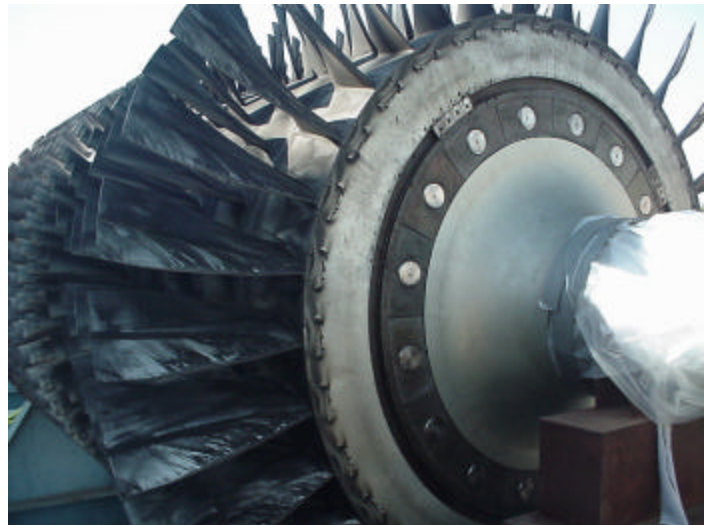
Figure 7 Contamination of the first stages of compression. Note the cleanness of the stub shaft.
