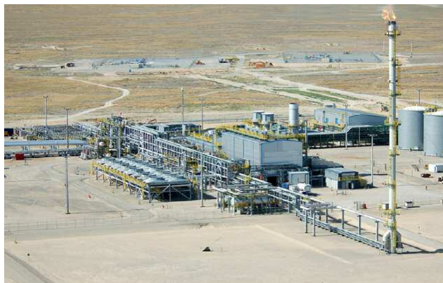
Figure 1. Tengiz Sour Gas Injection Compressor "Island" Station.
