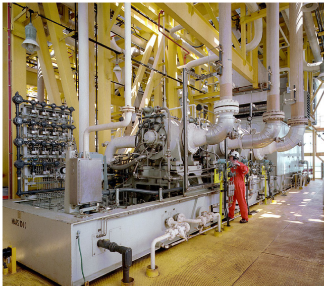
Figure 17. Offshore Gas Compressor Train. (Courtesy Solar Turbines Incorporated)
