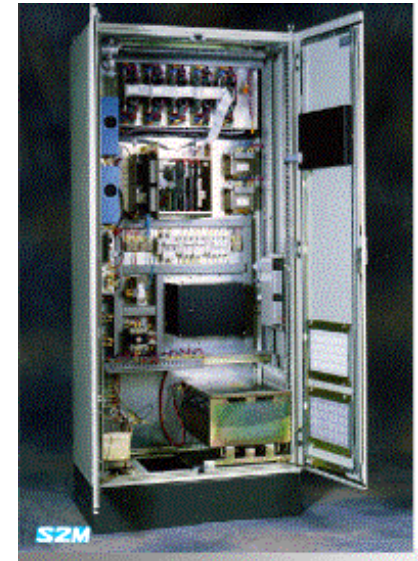
Active Magnetic Bearing Control Cabinet
