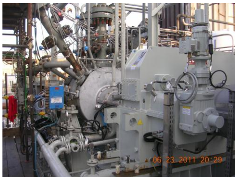
Figure 41. HP compressor casing instrumented as per ASME PTC10 requirements.
