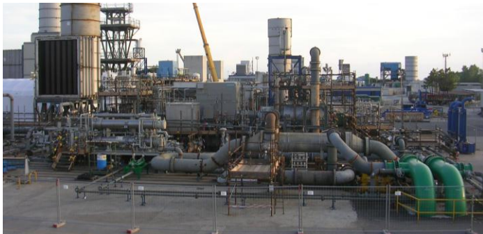
Figure 40. CO 2 Test bench and gas loop (Massa, Italy)
