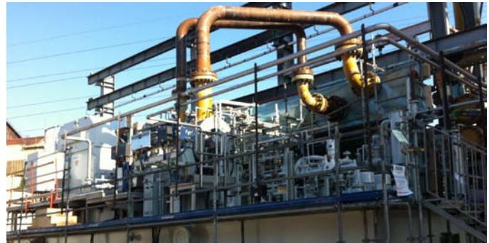
Figure 4: HP1 gas compressor package on the test facility, Le Creusot, France
