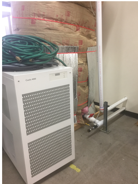
Figure 4.44: Tertiary reservoir, air-cooled chiller, and chilled water lines into the facility room
