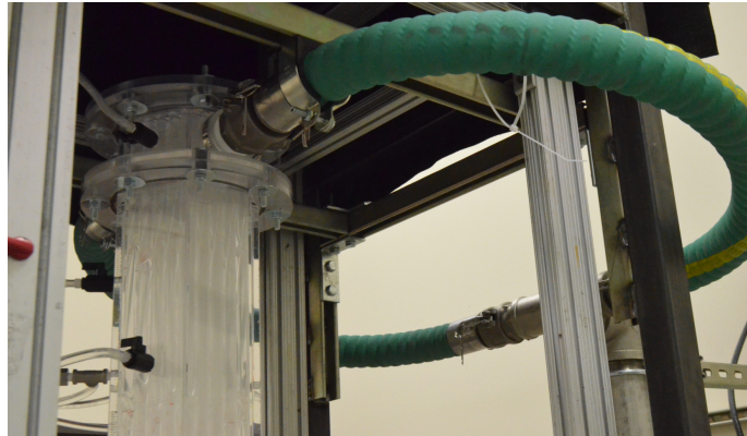
Figure 4.38: UHMWPE flexible hoses anchored to support structure
