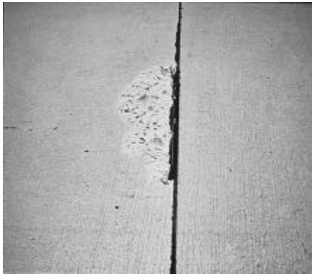
Figure 1 Beginning of a Spall (Fowler et al. 2008)
