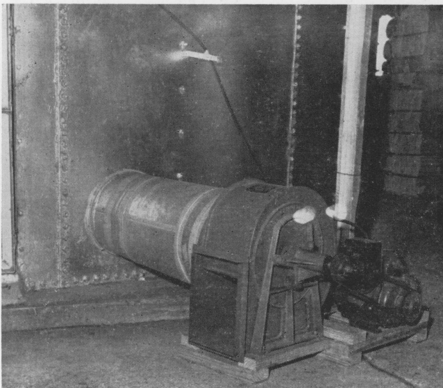
Figure 4. The centrifugal fan shown here was permanently installed to pull air through stored seed. This fan, operated by a 1-horsepower electric motor, supplied air at a rate of 5.4 cfm per minute per ton of cottonseed.
