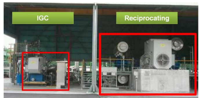
Figure 9. IGC and Reciprocating Compressor in Same BOG Application
