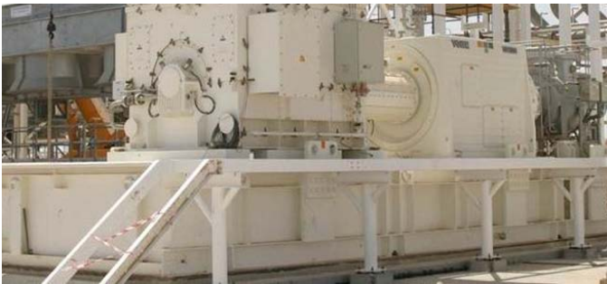
FIGURE 31: HYDRODYNAMIC VARIABLE SPEED PLANETARY GEAR IN COMPRESSOR TRAIN
