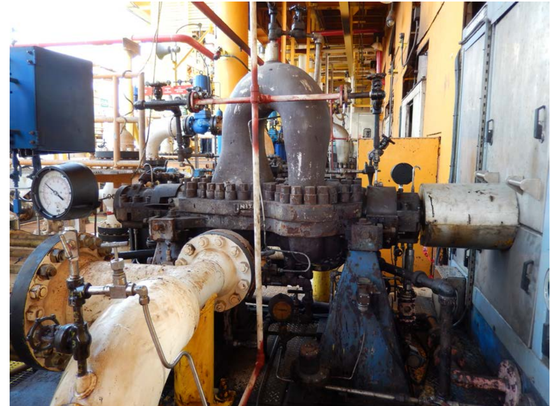
Centrifugal Pump with Shaft Guard On
