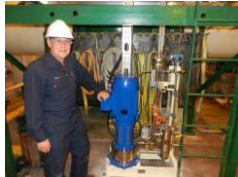
Figure 28: Installed booster skid
