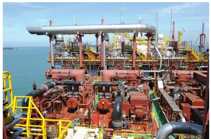
Figure 7. Three 24 MW condensing steam turbine generator sets on board the Peregrino FPSO.
