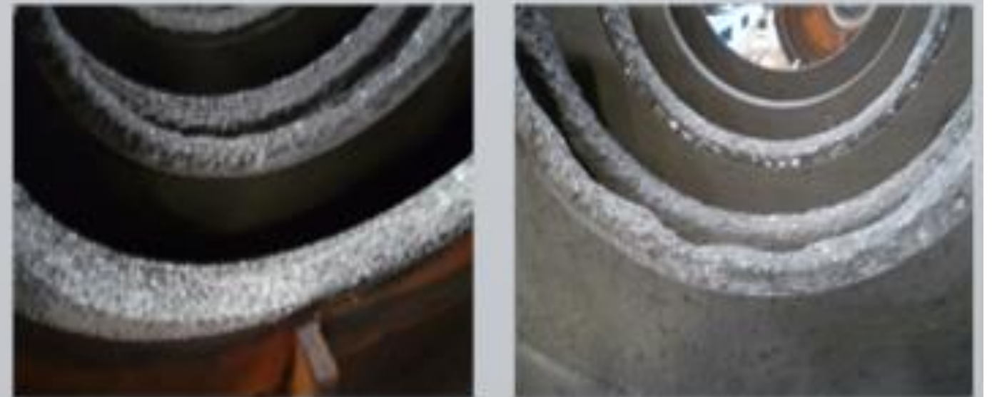
Impeller labyrinth corroded
