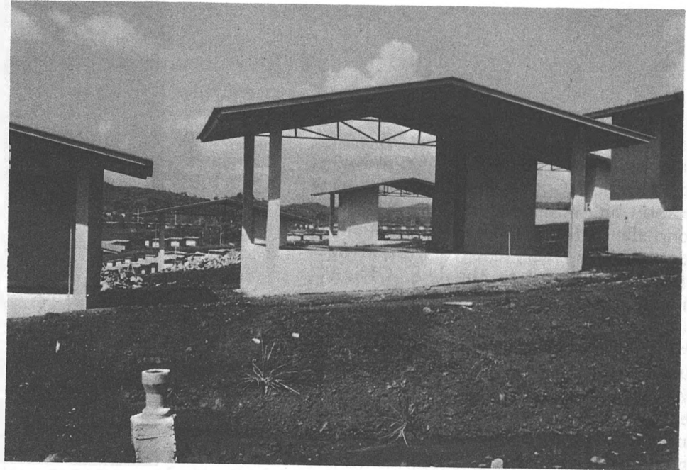
Roof-floor unit, soon to be completed by owners. As of 12/30/80, 250 of the 417 roof-floor units were enclosed, with the balance expected to be complete by 6/30/81.
