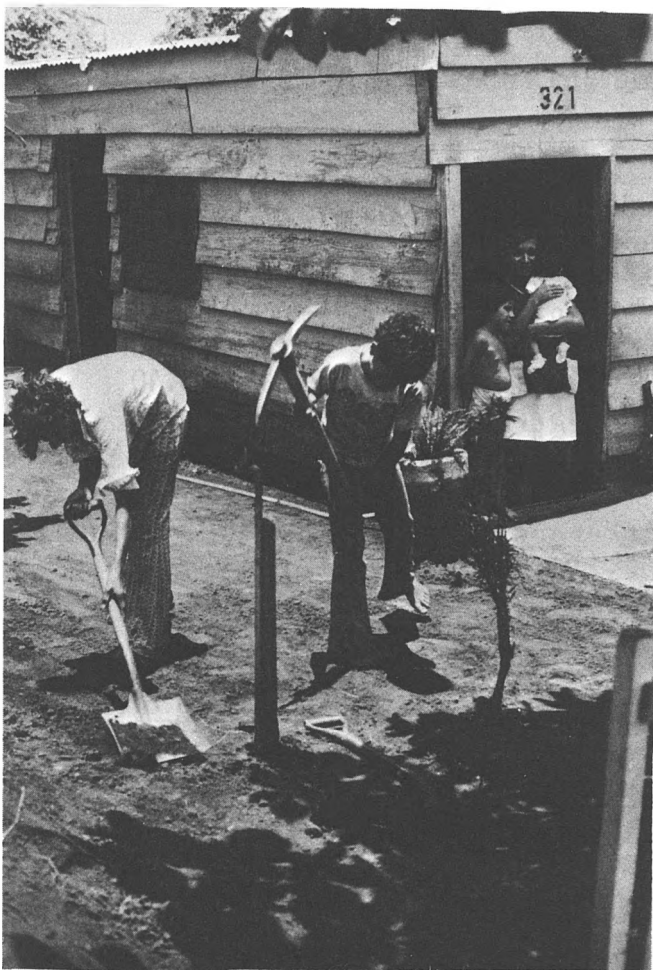
As part of an upgrading program, family is completing installation of water standpipe which brings potable water to their door.
