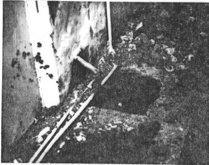
Figure 6: Latrine Drainpipe Emptying into Storm Drain
