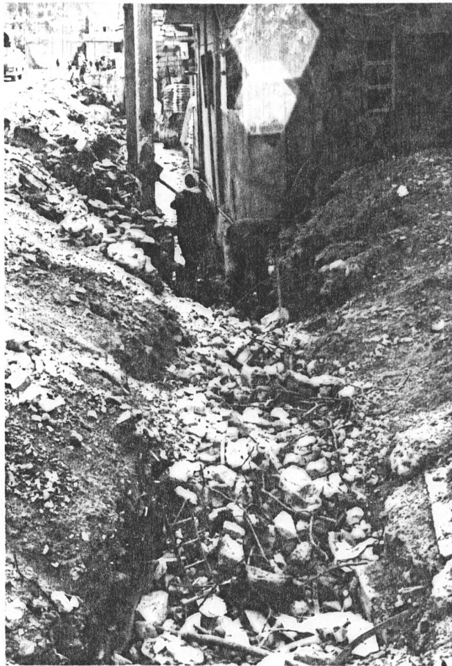
Figure 12: Clearing an Entrance to a Repaired House (Ayn al-Hilwah). Note the height of the road and regraded land adjacent to the house.
