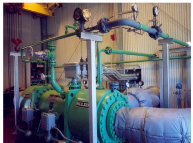
Figure 2: First Integrated Pipeline Motor-Compressor at Station 100 (USA), 1990
