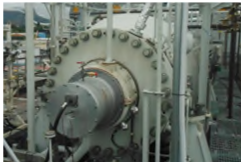
Figure 20 - Photo of the Magnetic Exciter used during the Lateral Stability Testing of Methane High Pressure Compressor
