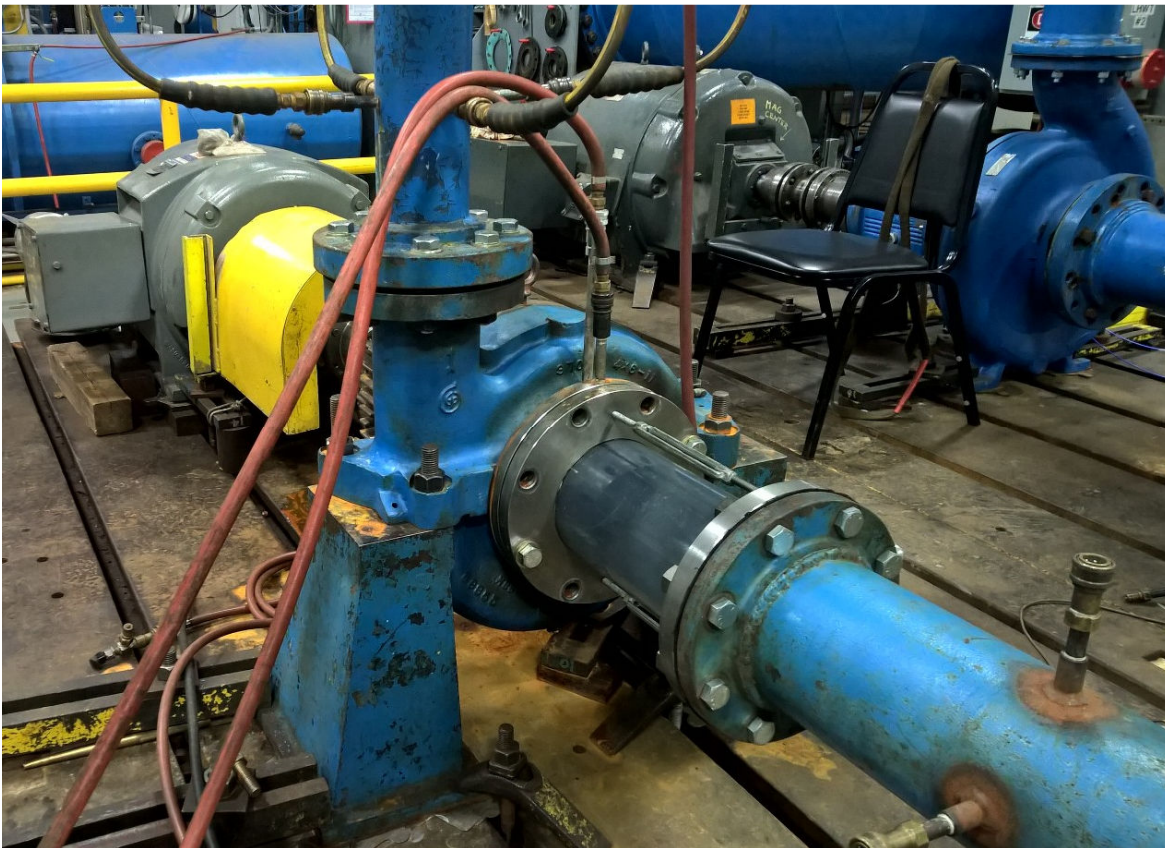
Figure 1: Pump installed in the test loop
