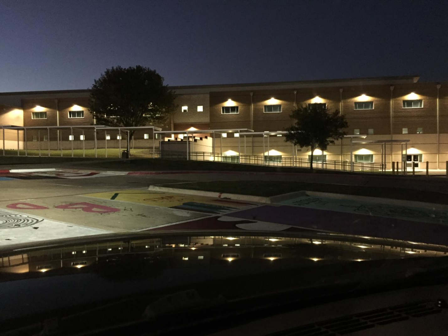
LED Wall Packs at Wylie High School
