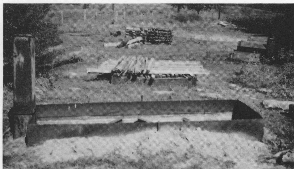
Figure 2. This vat for warm soaking posts in borax-water is placed over a trench. The sides and one end of the trench are sealed with dirt; the chimney is built of old ice cans.
