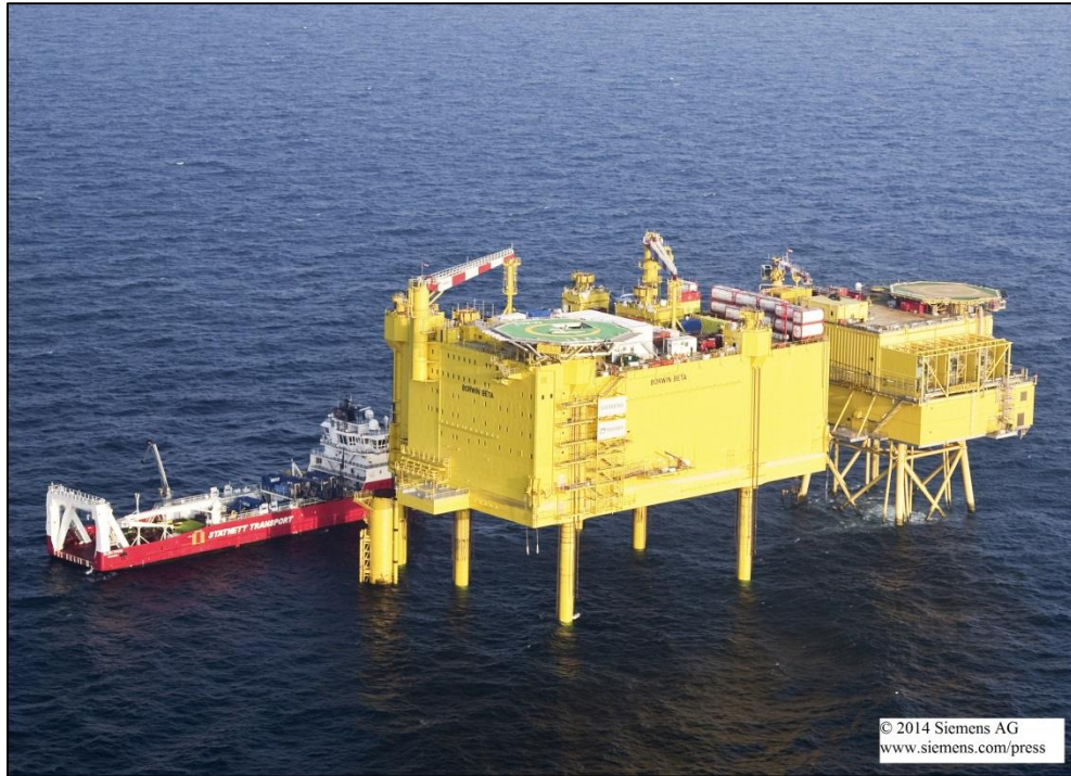
Figure 1-12: Example of an offshore HVDC converter station. Photo: Siemens AG 2014 [19]. Reused with courtesy of Siemens AG.
