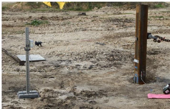
Figure 3-23: String potentiometer used for measuring lateral displacement
