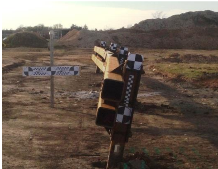
Figure 3-48: Permanent deflection of the piles and beams and barrier damage
