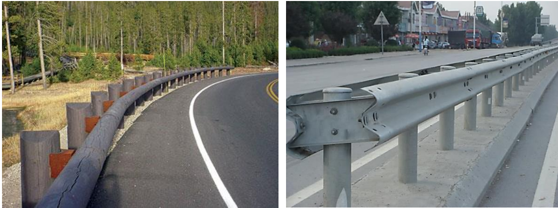
Figure 1-4: Typical roadside safety hardwares (FHWA publications)
