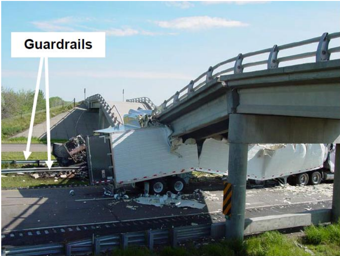
Figure 1-5: Collapse of I-80 bridge hit by tractor trailer, 2003 (El-Tawil, 2004, Photo Courtesy of NDOR)
