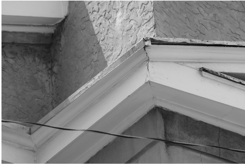
FIGURE 56. Image of cracking wood trim. (Photograph by the author)
