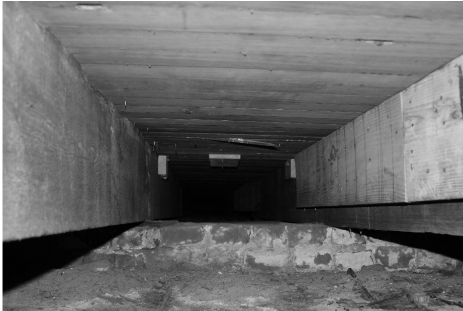
FIGURE 30. Wood beams in crawl space over brick grade beam of the First African Baptist Church (Photograph by the author)
