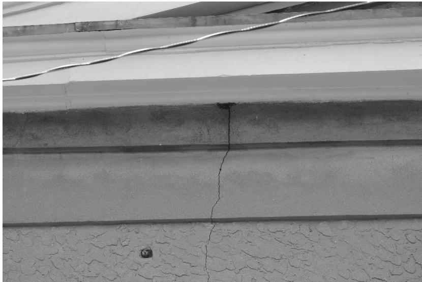
FIGURE 54. Image of cracking in the stucco finish. (Photograph by the author)
