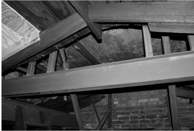
FIGURE 64. Image of steel structural members in the steeple of the church. (Photograph by the author)
