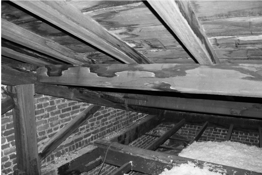
FIGURE 47. Image of wood purlins, using a birdnotch joint, supported by heavy timber structural members. (Photograph by the author)
