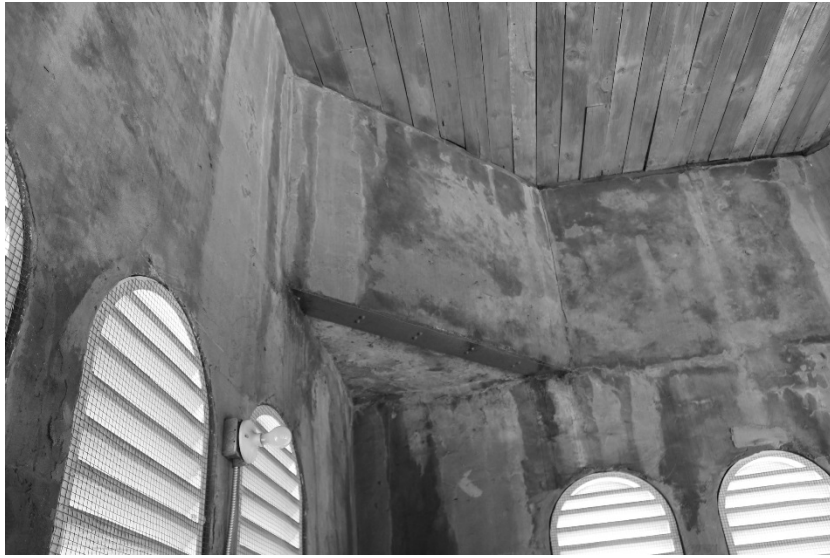
FIGURE 70. Image of the interior of the existing steeple. (Photograph by the author)
