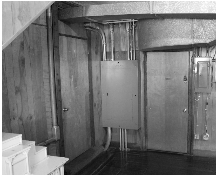
FIGURE 78. Image of wall mounted electrical panelboards (Photograph by the author)
