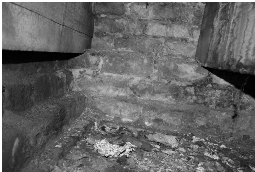
FIGURE 29. Wood beams in crawl space framing into perimeter brick foundation at the First African Baptist Church (Photograph by the author)
