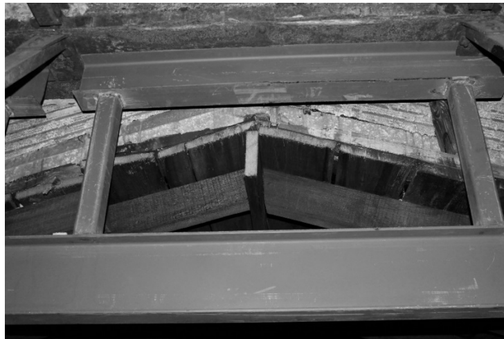
FIGURE 65. Image of steel structural members in the steeple of the church. (Photograph by the author)
