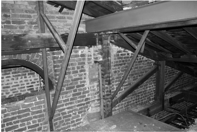
FIGURE 66. Image of steel structural members in the steeple of the church. (Photograph by the author)
