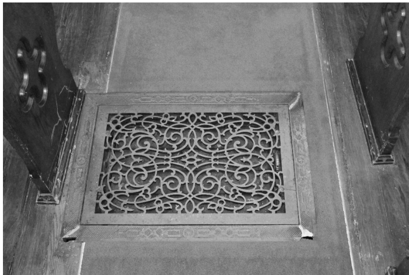
FIGURE 77. Image of HVAC floor grate in the sanctuary. (Photograph by the author)
