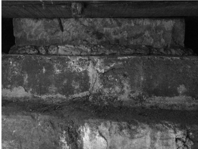
FIGURE 38. Stone atop masonry step footing supporting pipe column above, at the First African Baptist Church (Photograph by the author)
