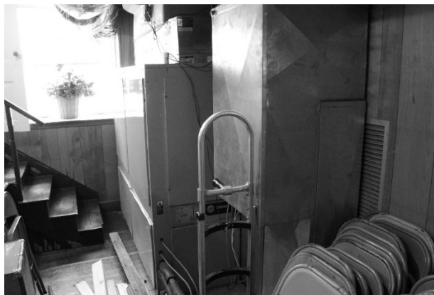
FIGURE 75. Image of one of the HVAC units. (Photograph by the author)
