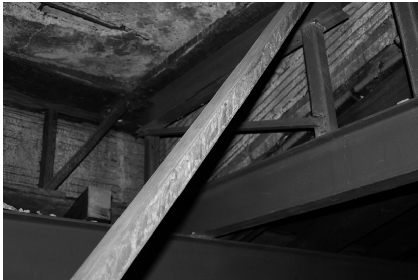
FIGURE 67. Image of steel structural members in the steeple of the church. (Photograph by the author)
