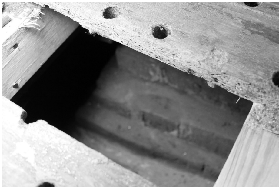
FIGURE 31. Opening in floor with view of column masonry step footing of the First African Baptist Church (Photograph by the author)
