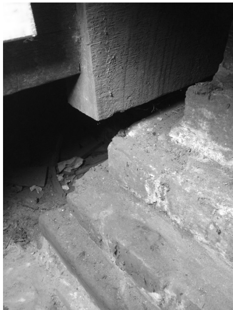
FIGURE 39. Profile of masonry step footing and wood beams in crawl space at the First African Baptist Church (Photograph by the author)
