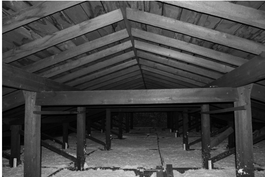
FIGURE 46. Image of heavy timber structural members framing the roof of the church building. (Photograph by the author)
