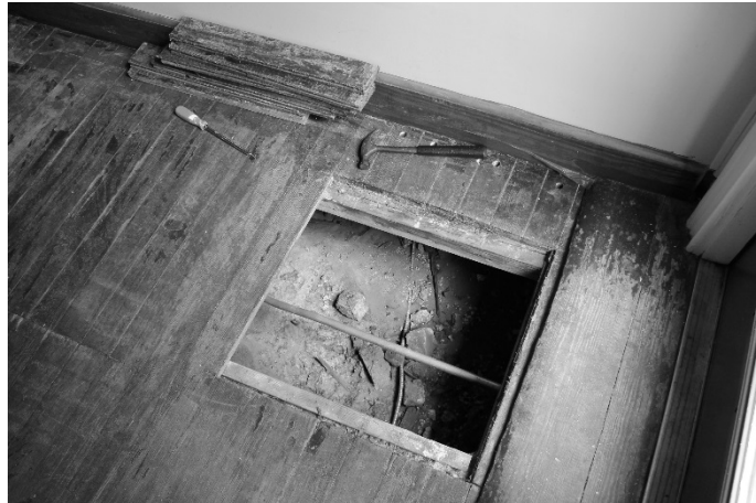
FIGURE 81. Image of floor access opening to crawl space (Photograph by the author)
