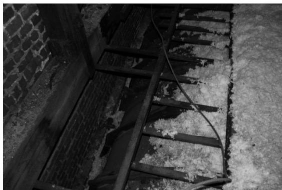
FIGURE 85. Image of the stamped metal ceiling and framing from the attic. (Photograph by the author)
