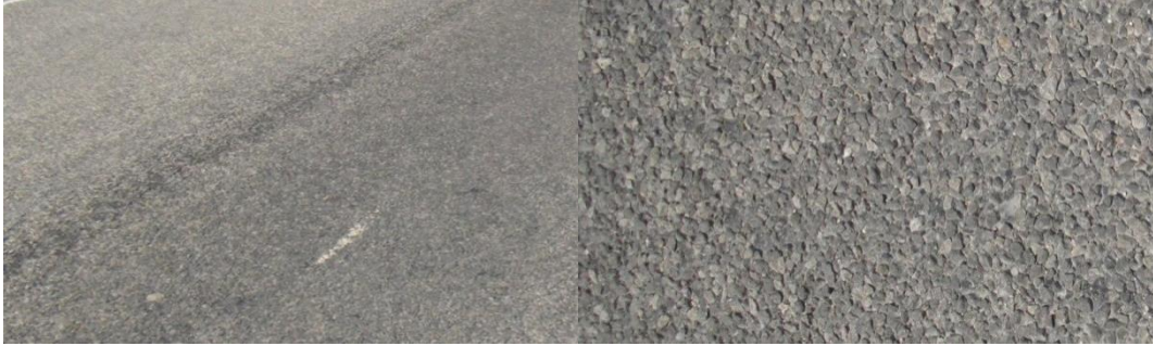
Figure 24. Example of Adequate Performance—HS SJT-b 1 Year after Construction.
