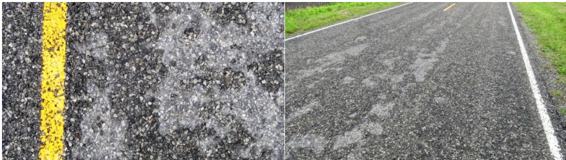
Figure 25. Example of Inadequate Performance—HS CRP-c 1 Year after Construction.
