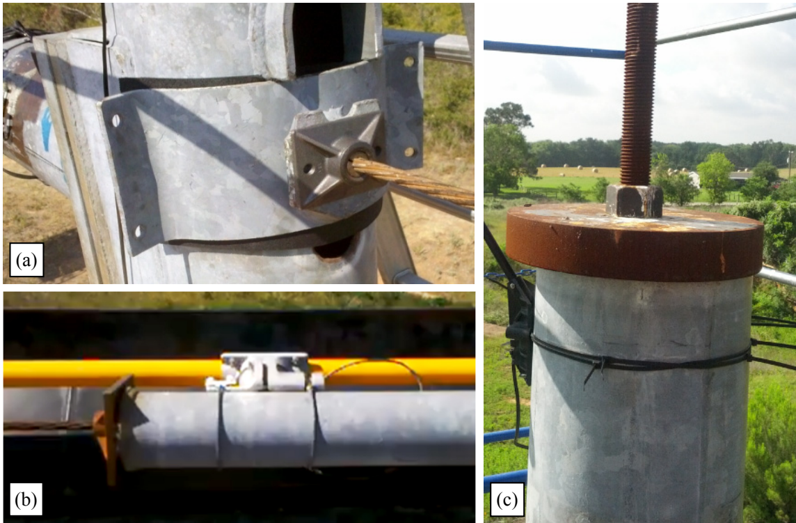
Figure 7-4. Photos depicting installation of the proposed arm PT system from the (a) backside of the arm-pole connection and (b) mast arm end, and (c) the pole PT system from atop the pole.
