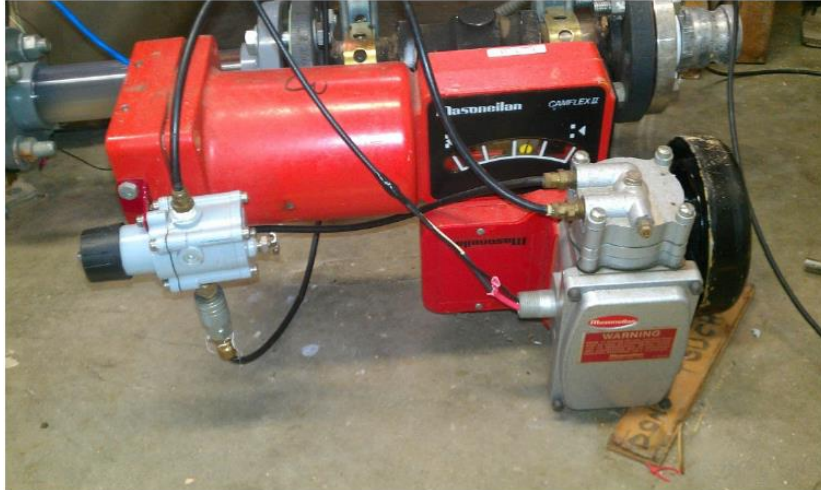
Figure 8: Masoneilan Dresser Varimax 3000 Series Control Valve
