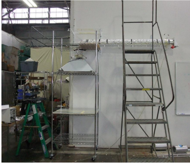
Figure 15. Case 1 (Flexible Duct) Pressure Measurement Test Setup
