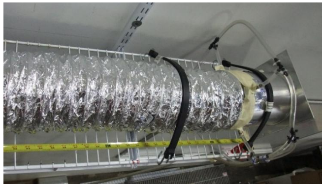
Figure 22. Flexible Duct Fastened to Shelving with a Rubber Attachment
