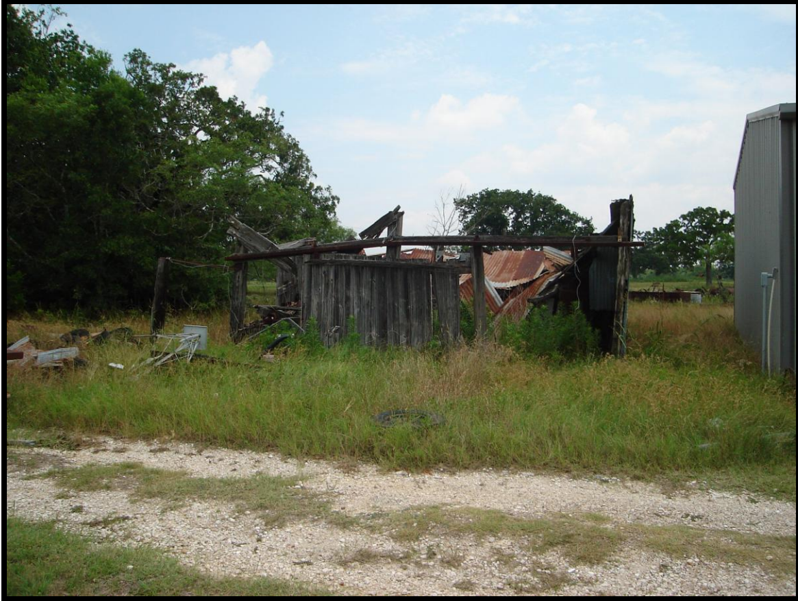
Structure F (collapsed pole barn)
