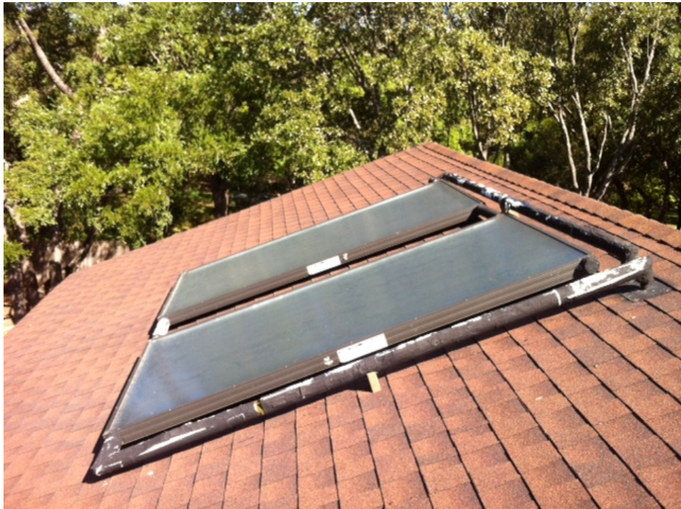
Fig. I.2. The solar collector panels.
