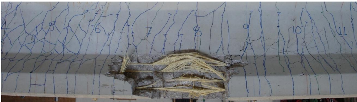
Figure 5-4. Tendon Rupture at the Bottom Flange as the Failure Mode.
