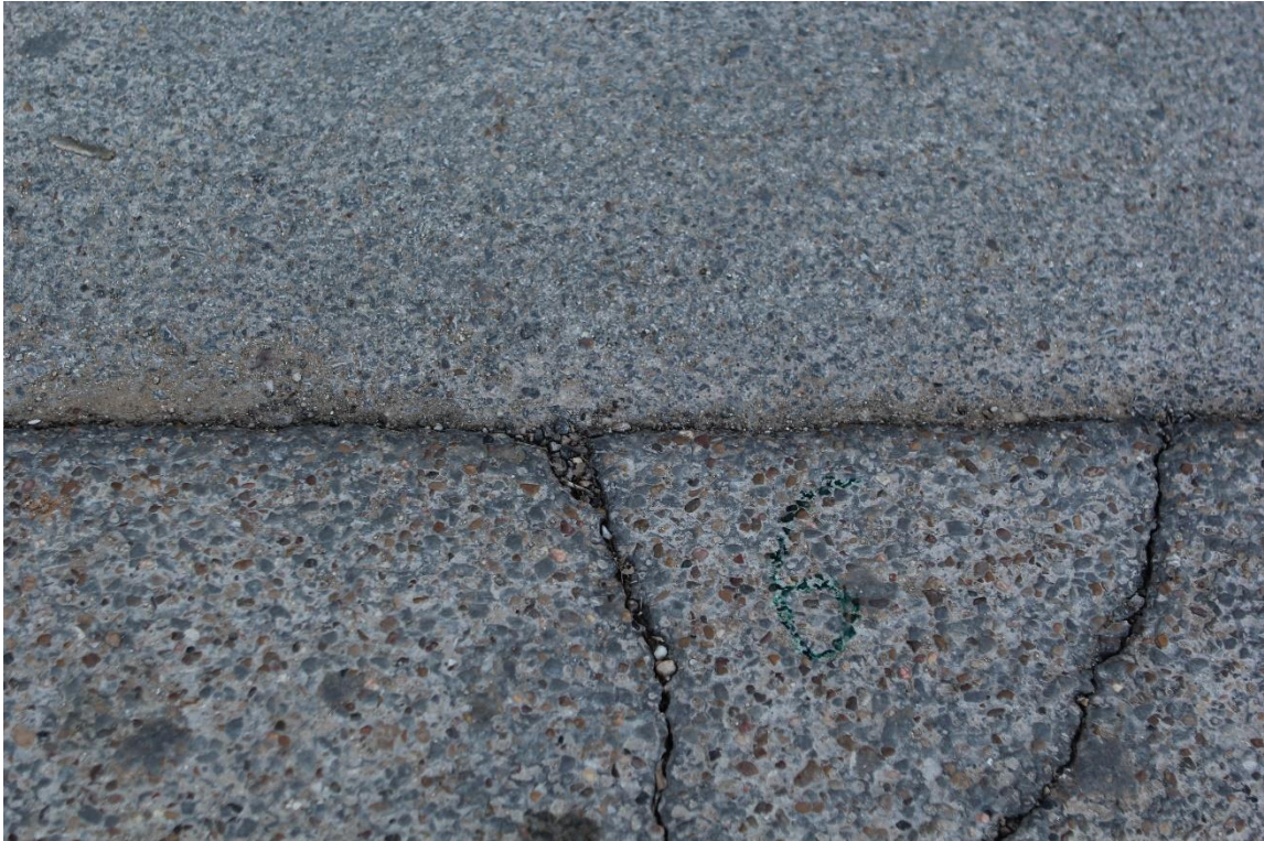
Figure 21. Photograph crack No.6
