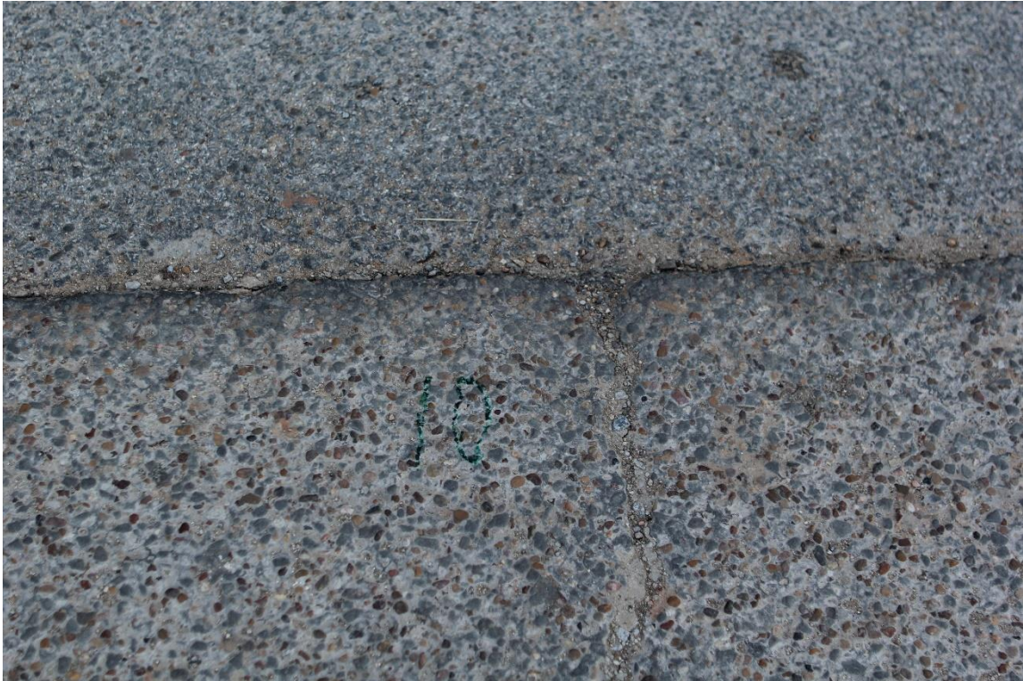
Figure 25. Photograph crack No.10
