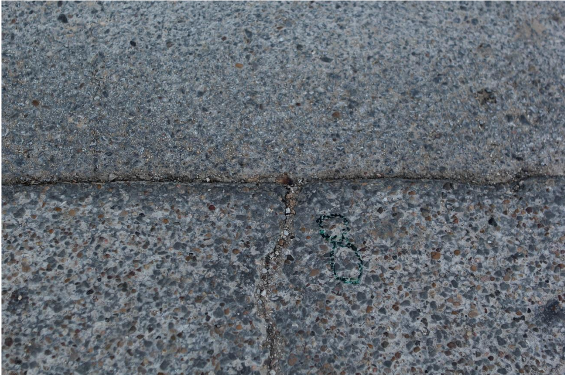
Figure 23. Photograph crack No.8
