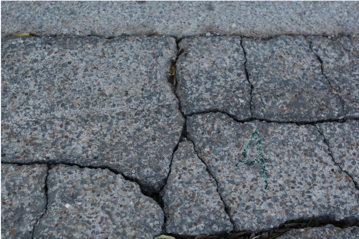
Figure 19. Photograph crack No.4
