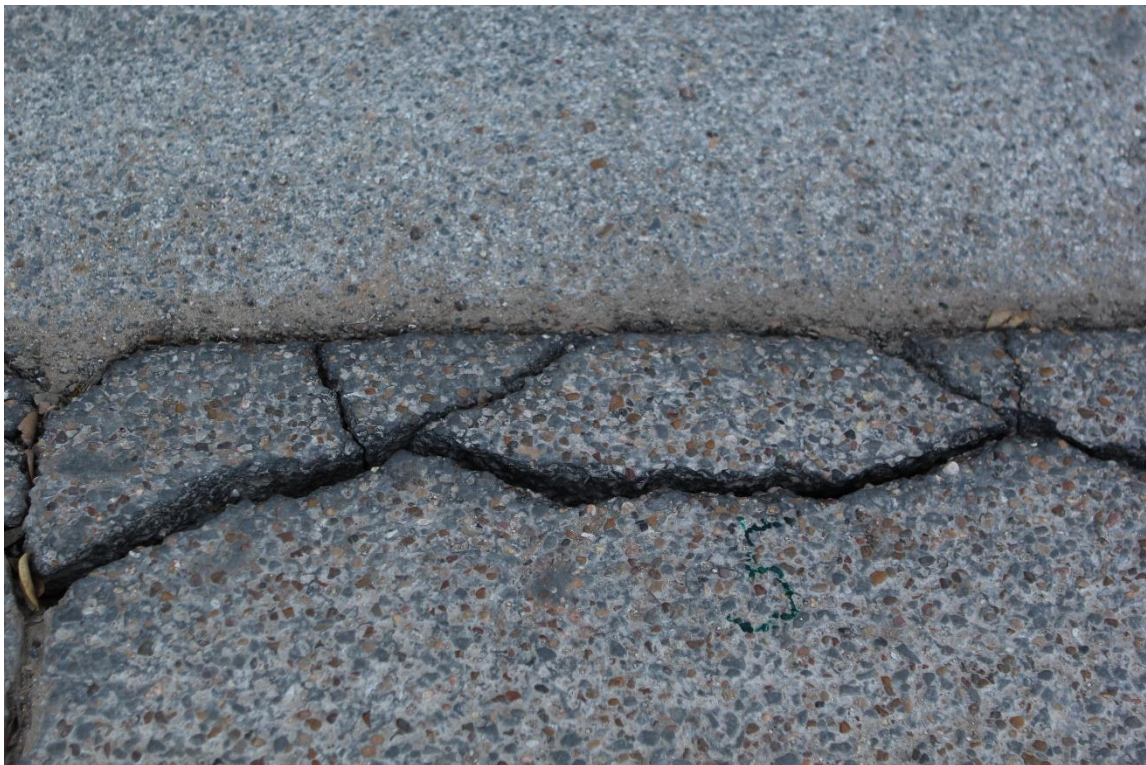
Figure 20. Photograph crack No.5
