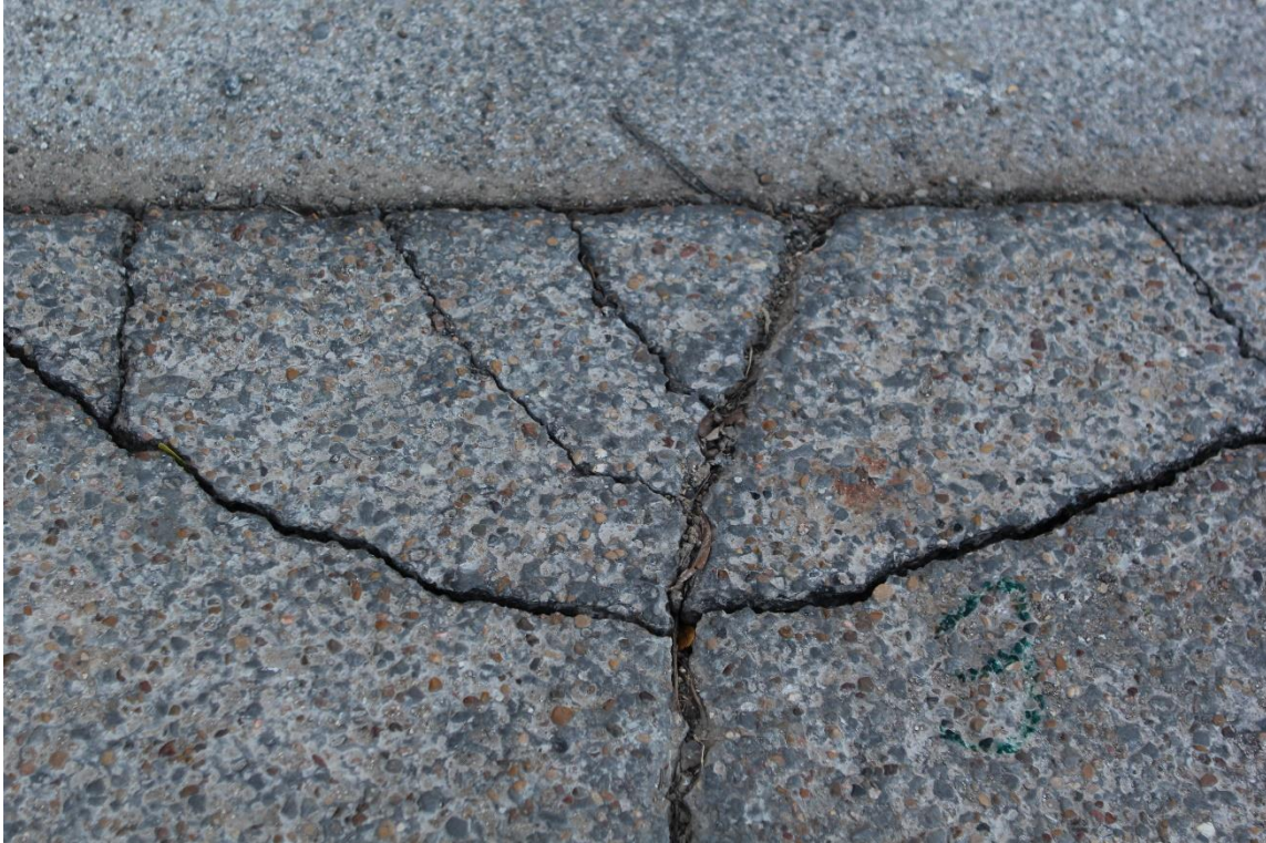
Figure 18. Photograph crack No.3
