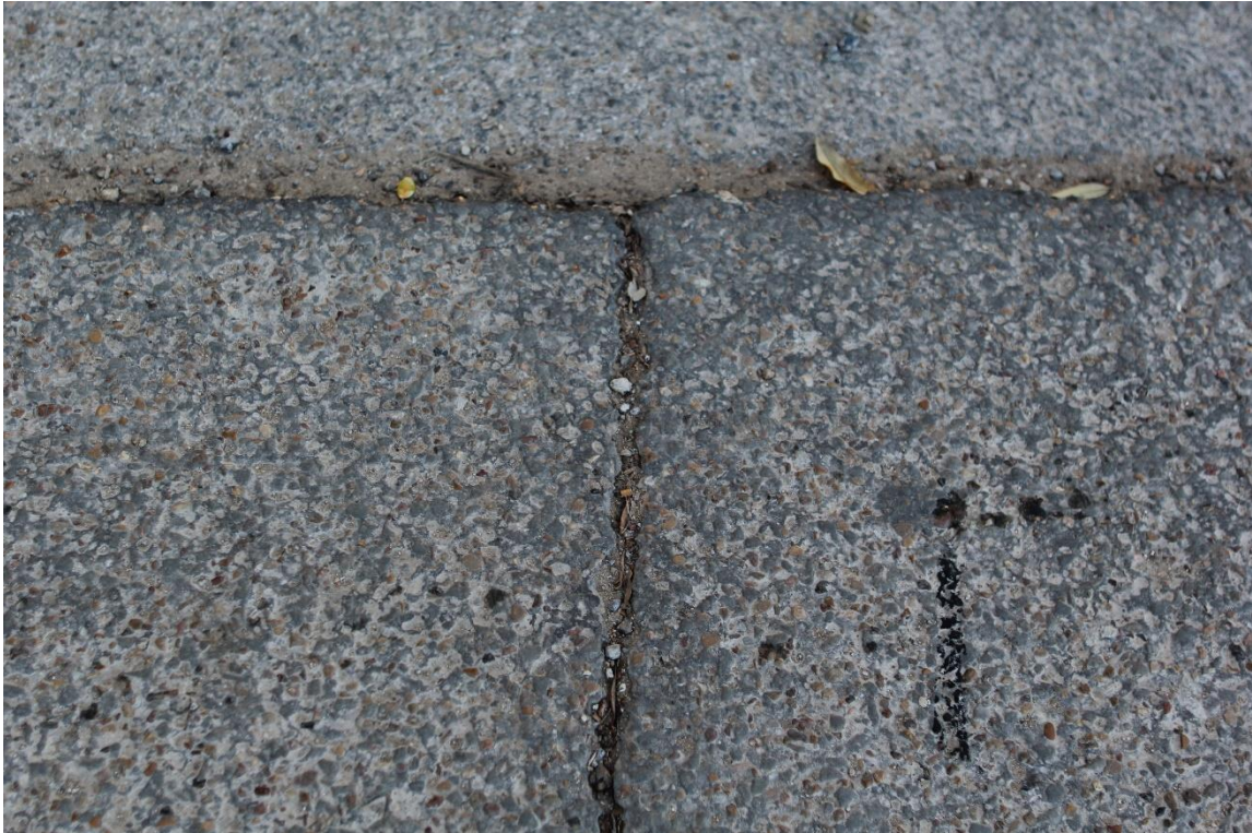
Figure 16. Photograph crack No.1
