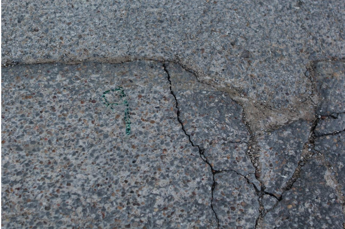
Figure 24. Photograph crack. No.9
