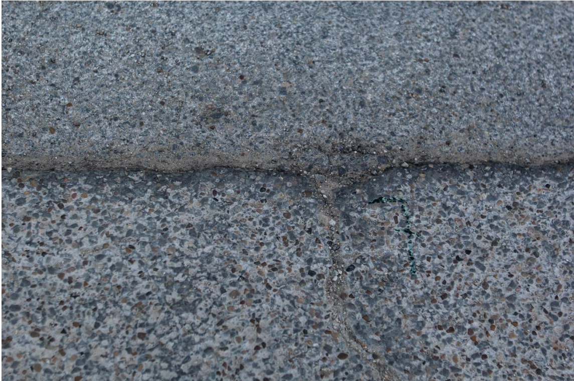
Figure 22. Photograph crack No.7
