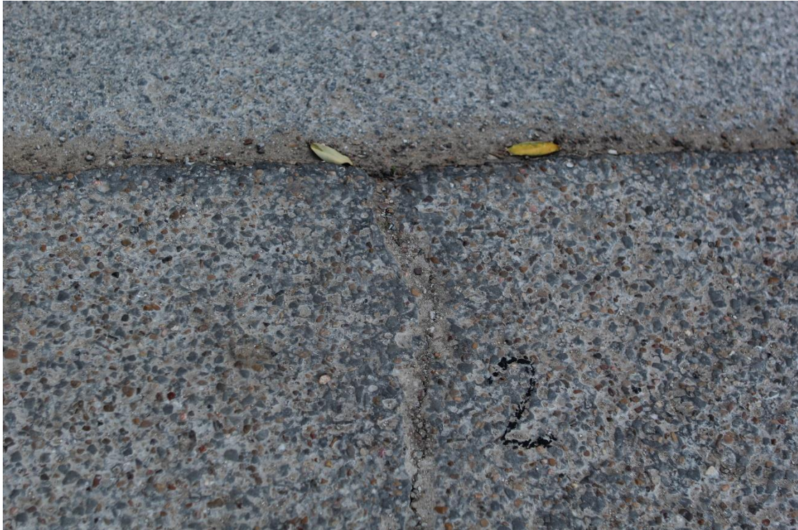
Figure 17. Photograph crack No.2
