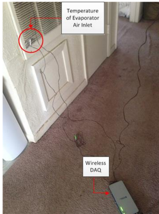
Figure 30: Temperature Sensor for Return Air Temperature and the Wireless DAQ at the Indoor Unit
