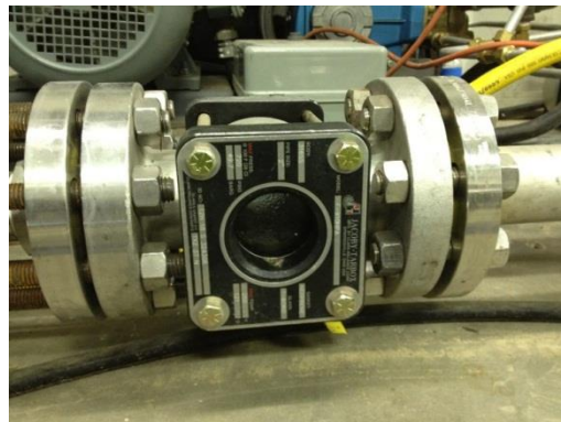
Figure 3-10: Air line sight glass
