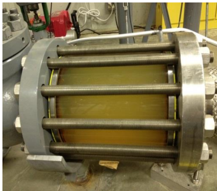
Figure 3-9: Water line sight glass
