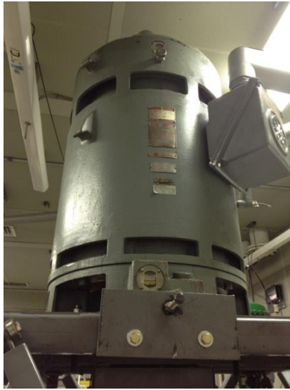
Figure 3-4: 250 hp AC Motor
