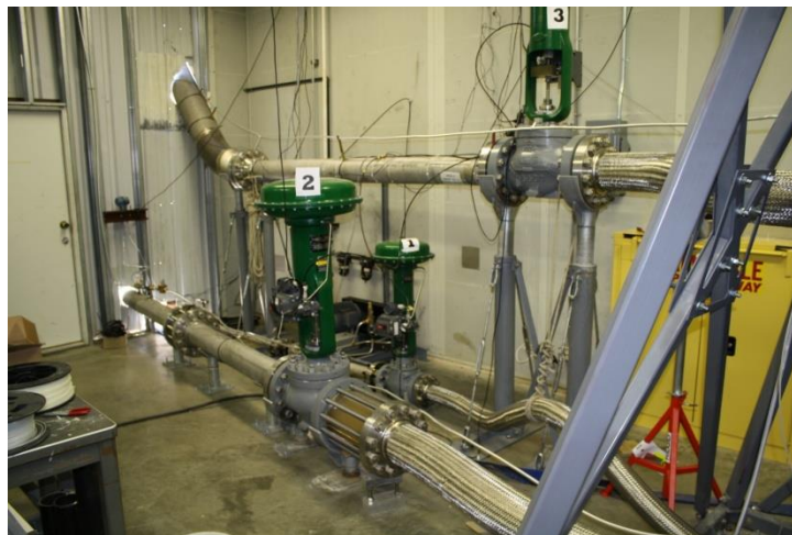
Figure 3-5: Control Valves, 1) Air control Valve, 2) Water control valve, 3) Outlet control valve
