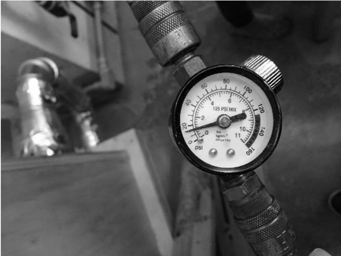
Figure 26. Pressure Gauge for Inflow Air
