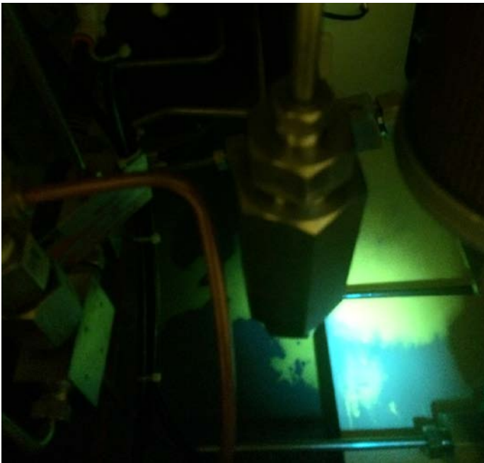
Figure 36: Leaking from Air Operated Valve
