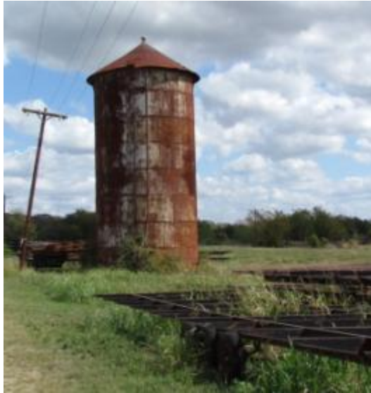
Figure 215 Camp Hearne Water Tower in 2011
